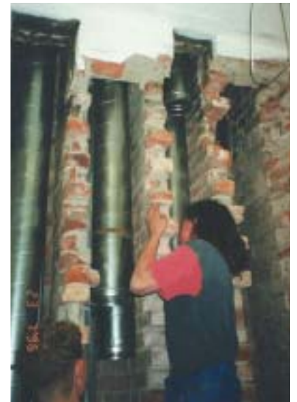
Foto: Vertical air ducts were built into the old ventilation shafts
