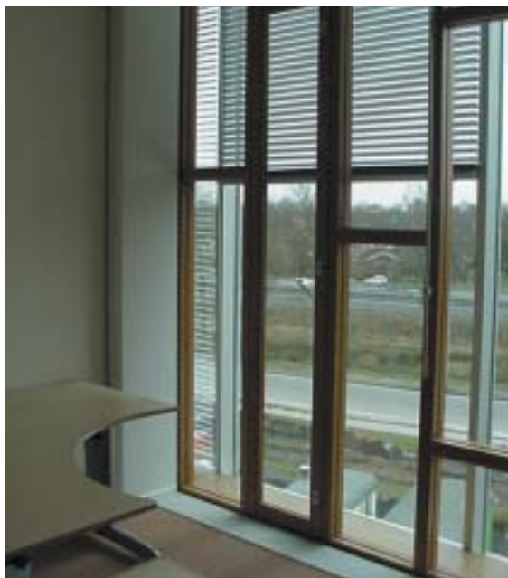
Fig 2 Climate facade at the ICT Business Centre Groningen Photo: BV Technical Management (TM).
