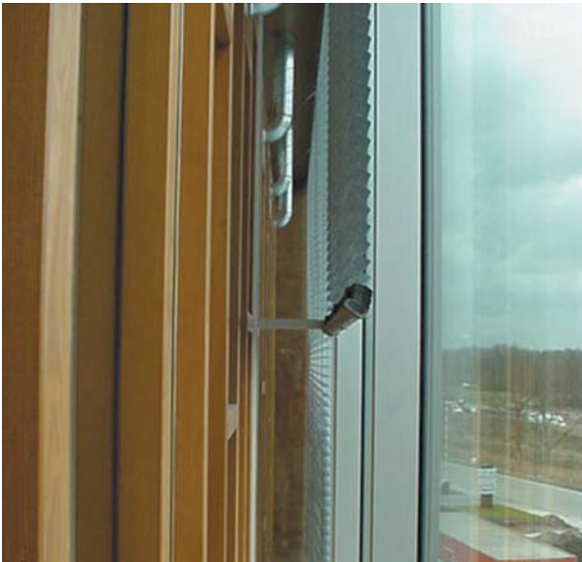
Fig 24 Climate facade with sun-blinds installed in the cavity.
