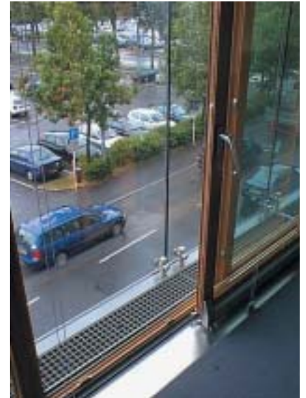
Fig 9 Banque Générale, Limpertsberg in Luxembourg; Double-skin facade of the 6-storey office building. Photo: Goblet & Lavandier
